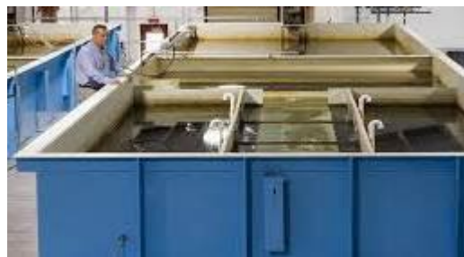
Fig 1. Package Water Plant.
